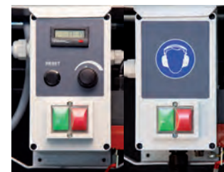
Different control units
