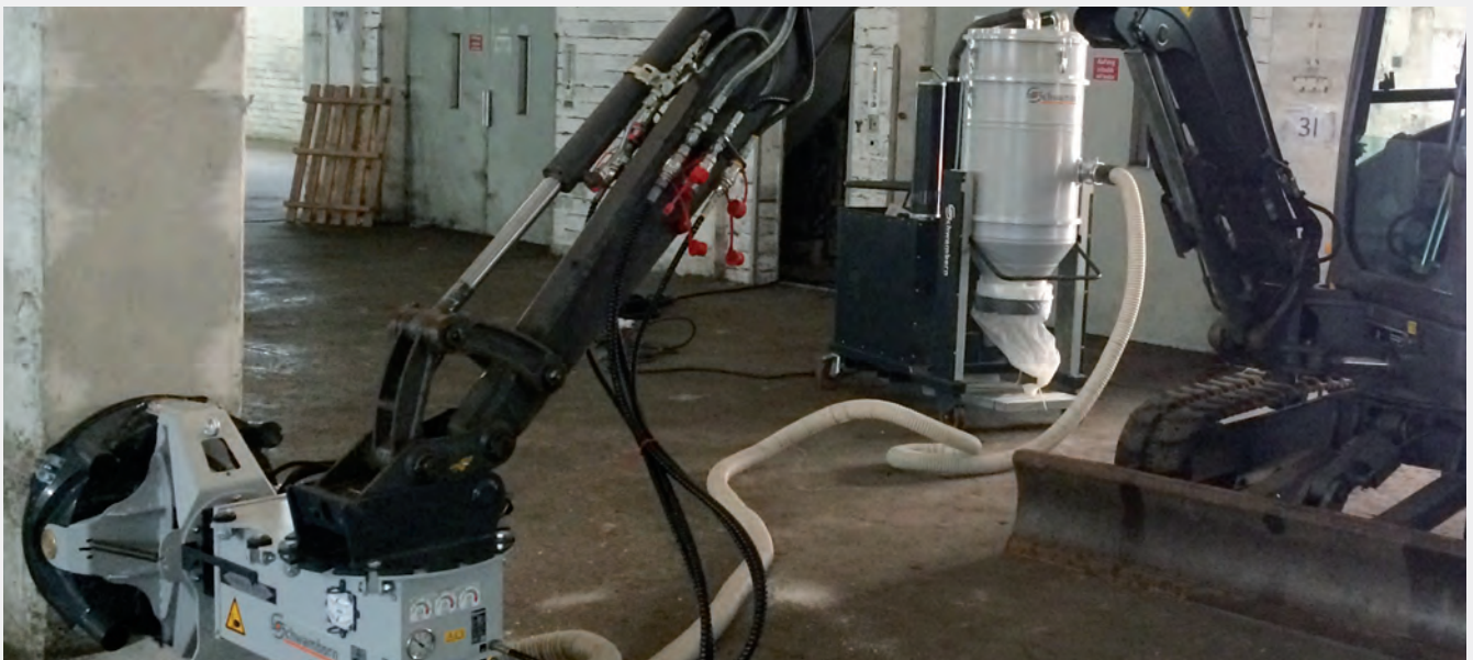
There are four suction nozzles on the sanding head of the WDS, enabling suction from multiple points. An advantage with contaminated material.
